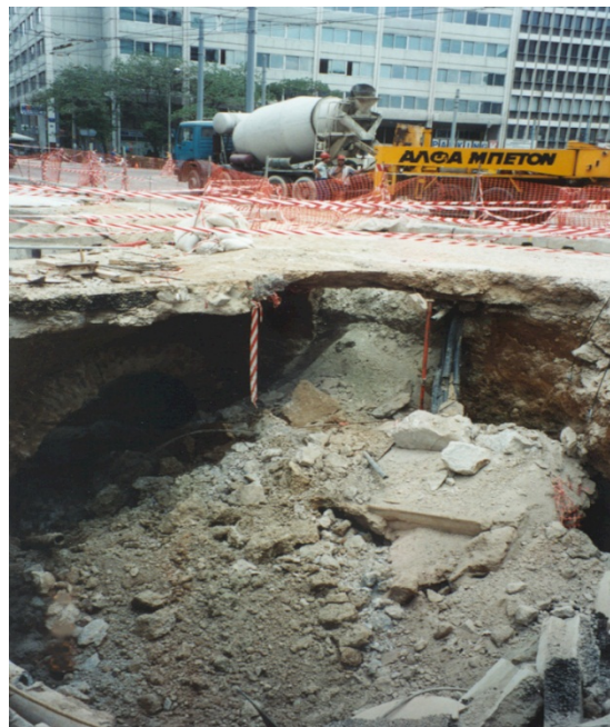
Figure 3. Significant over-break failure at Aghiou Konstantinou street. Athens Metro project.
