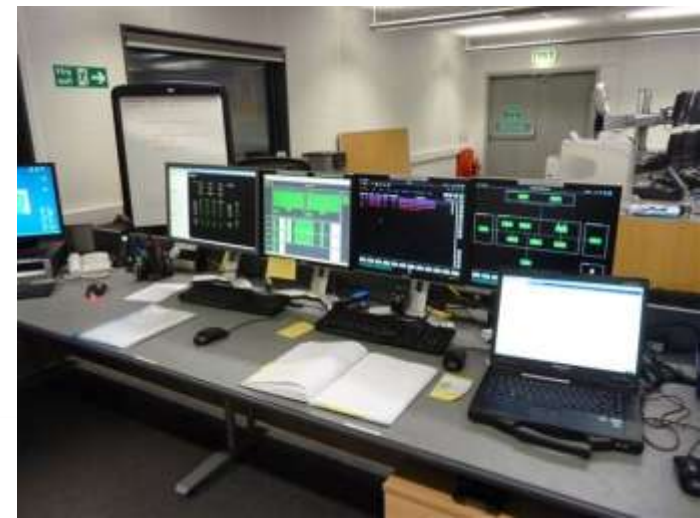
Box Technicians desk
